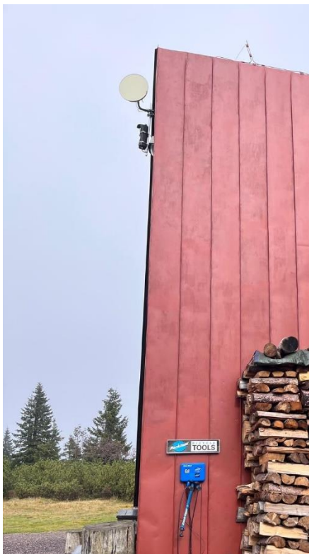
The installed sensor at one building of KRNAP – National Park Krkonose.
